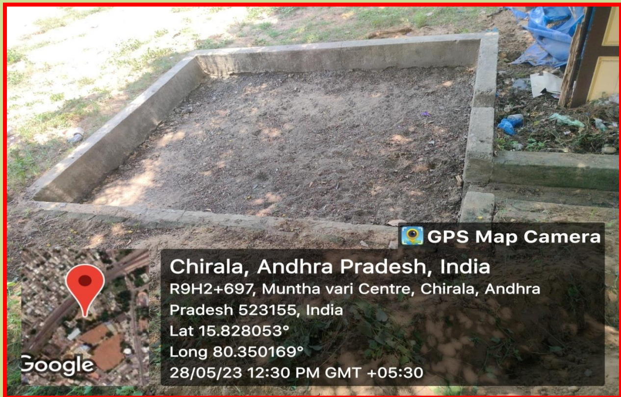
Rain water harvesting pit at Seminar Hall in the campus
