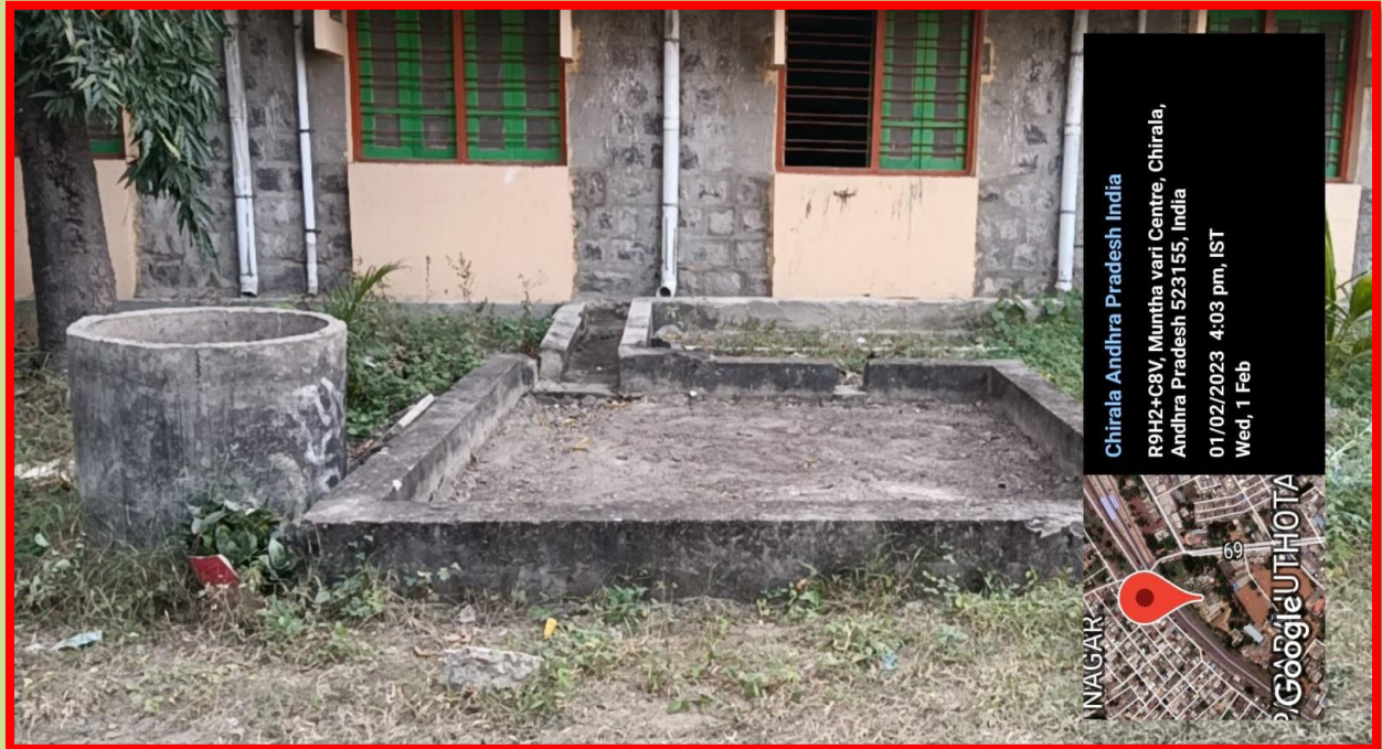
Rain water harvesting pit at Main Building in the campus
